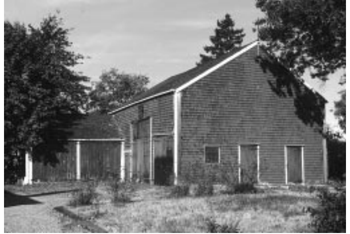
DHS needs more money to fix the barn roof, with the hope of stabilizing the structure for future restoration.
